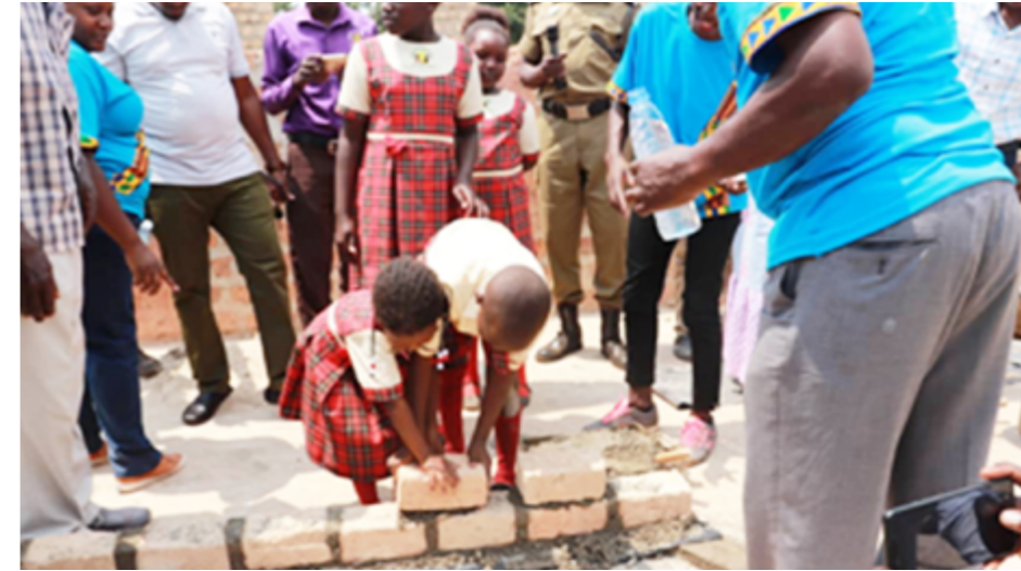
Pupils from Kings Norton school laying bricks as sign of setting up the walls with the help of Eng. Charles
