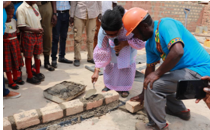
The guest of honor Dr. Thelma laying bricks as sign of setting up the walls with the help of Eng. Charles”.
